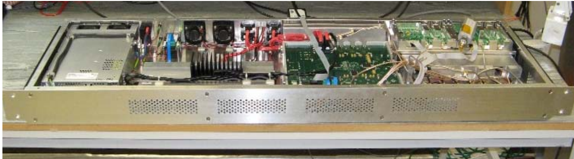
Figure 7. Rack Unit with Digital Transceiver and RF Up- and Down-Converters
